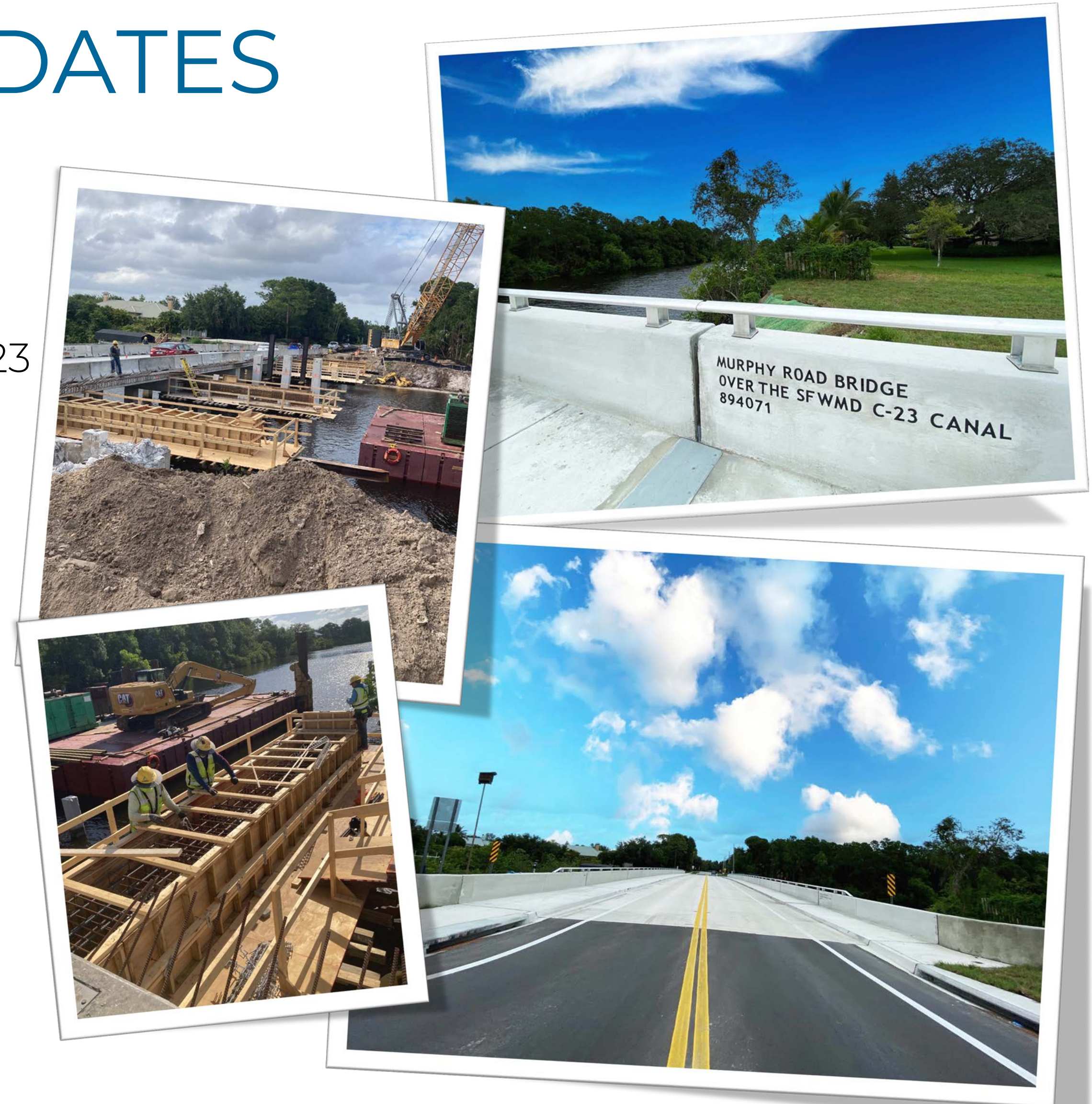
Murphy Bridge Road
