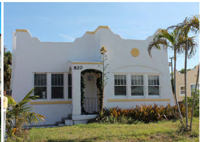
Articulated parapet on a flat roof on house in Lake Worth Beach, FL
